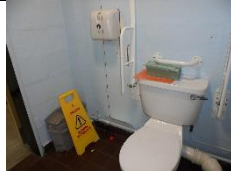
Bin and sign are in the way of a wheelchair user side transfer onto the toilet and paper dispenser too high
