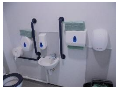
Toilet roll resting on grab bar restricts access
