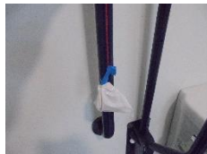
Emergency alarm cord should reach all the way to the ground
